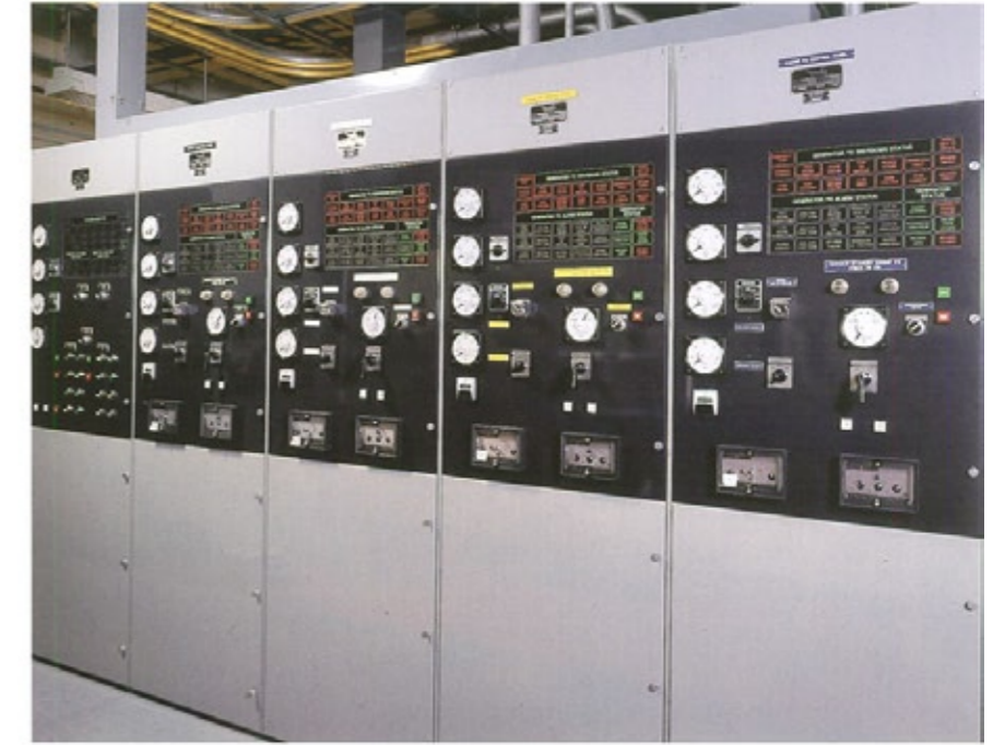
ENGINE GENERATOR PARALLELING CONTROLS
